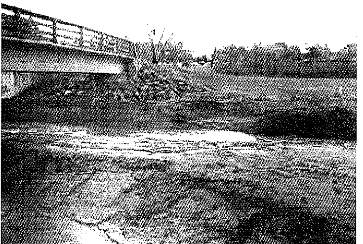
Sedimentation under a bridge
