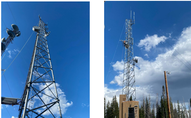
Photos on the left show construction of the new tower at Buffalo Pass nearing completion. Antennas have been moved from the temporary tower to the new tower and the temporary tower has been removed from the site and returned to Douglas County.
