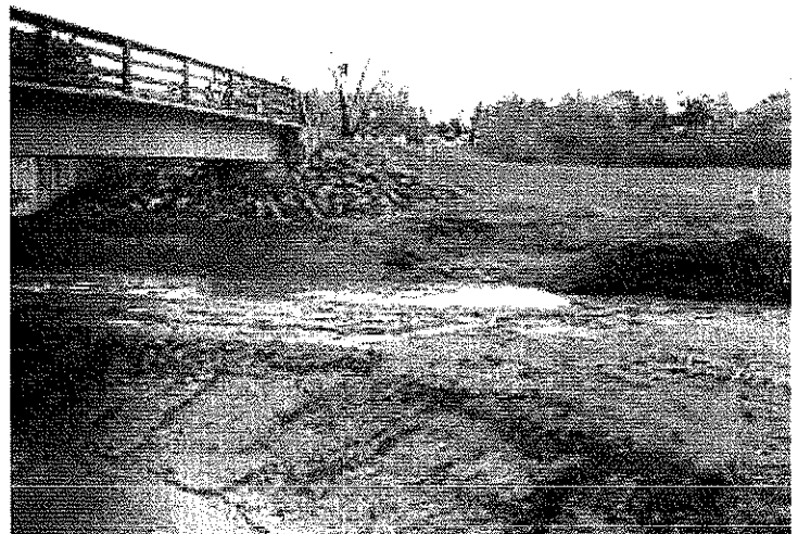
Sedimentation under a bridge
