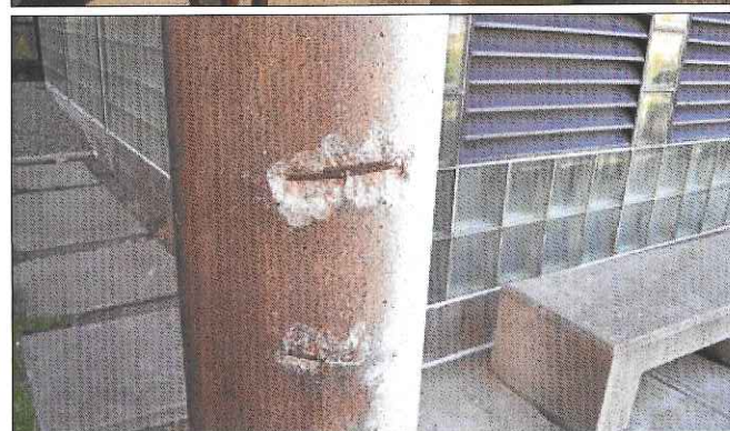
Deteriorating Building Structure
