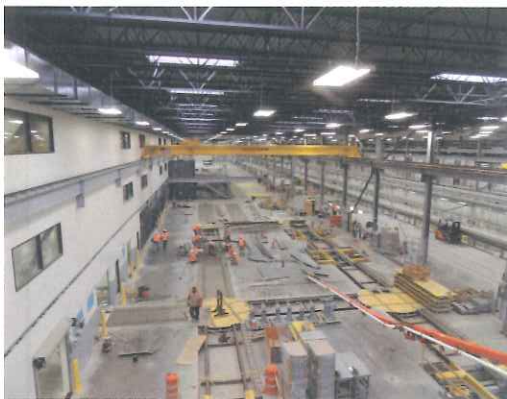
Up to 80 electric rail cars can be serviced in this massive facility.
