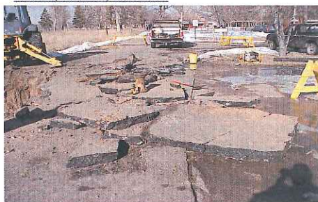
Water Main Break
