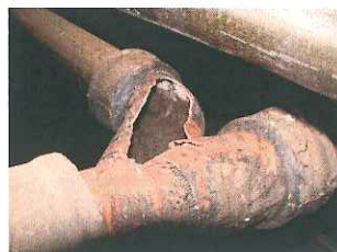
Sewer line deterioration
