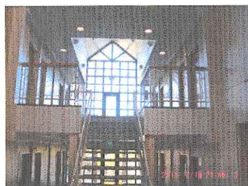
Lookout Mountain Youth Services Center Condition Pre-mitigation
