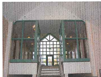
Lookout Mountain Youth Services Center Condition Post-mitigation
