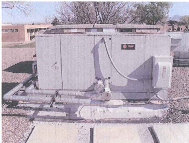
Photo 1 – Typical Rooftop HVAC Unit.
