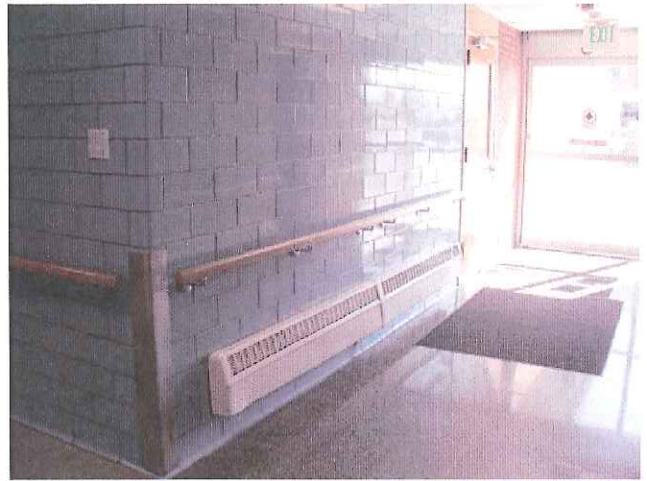
Photo 8 – Entry vestibule baseboard heating unit.
