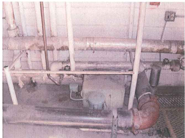
Photo 2 – Steam Condensate return pump
