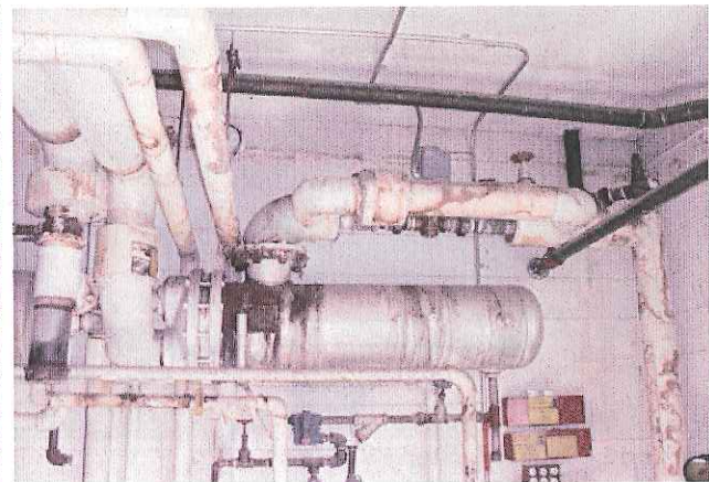
Photo 6 – Steam-to-Water Heat Exchanger for building heating water.
