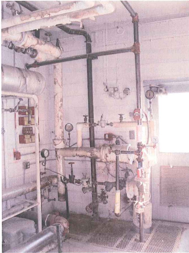
Photo 7 – Steam piping entry with insulation.
