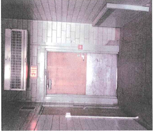
Code, Safety and Functional Deficiencies
