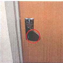
Colorado Mental Health Institute at Ft. Logan, F-Cottage Door Hardware - After Mitigation
