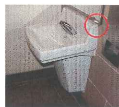
Colorado Mental Health Institute at Ft. Logan, F-Cottage Sink and Faucet - After Mitigation
