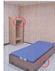
Colorado Mental Health Institute at Pueblo, Bldg. 116 Sleeping Room - Removed ventilation duct covers, replaced curtains, replaced dangerous furniture - After Mitigation
