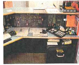
Gilliam control panel
