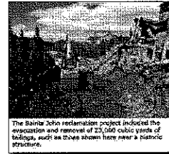
The Saints John reclamation project included the excavation and removal of 23,000 cubic yards of tailings, such as those shown here near a historic structure.
