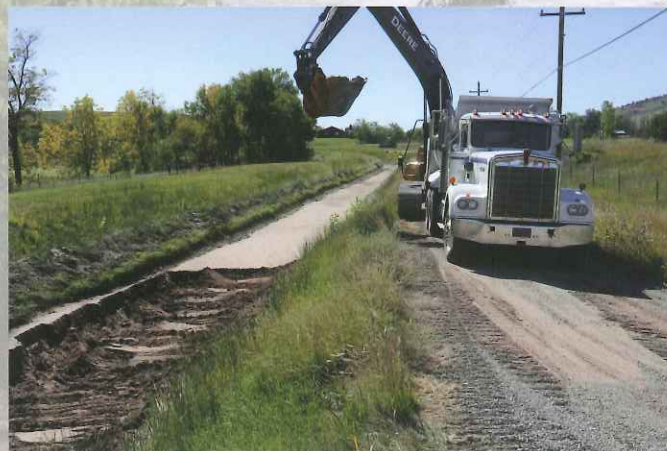
CLOCKWISE FROM TOP LEFT: Grading the eroded lining of the Boulder Feeder Canal north of the Left Hand diversion structure; cleaning up the Left Hand diversion structure on the BFC; removing debris from the St. Vrain Supply Canal outlet structure; removing silt from the flooded BFC just east of Highway 36 in Lyons
