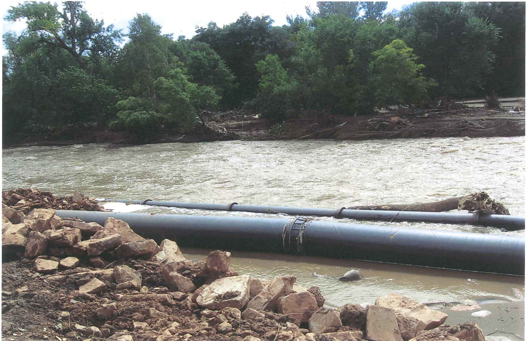
Loveland - Drinking Water Line Exposed
