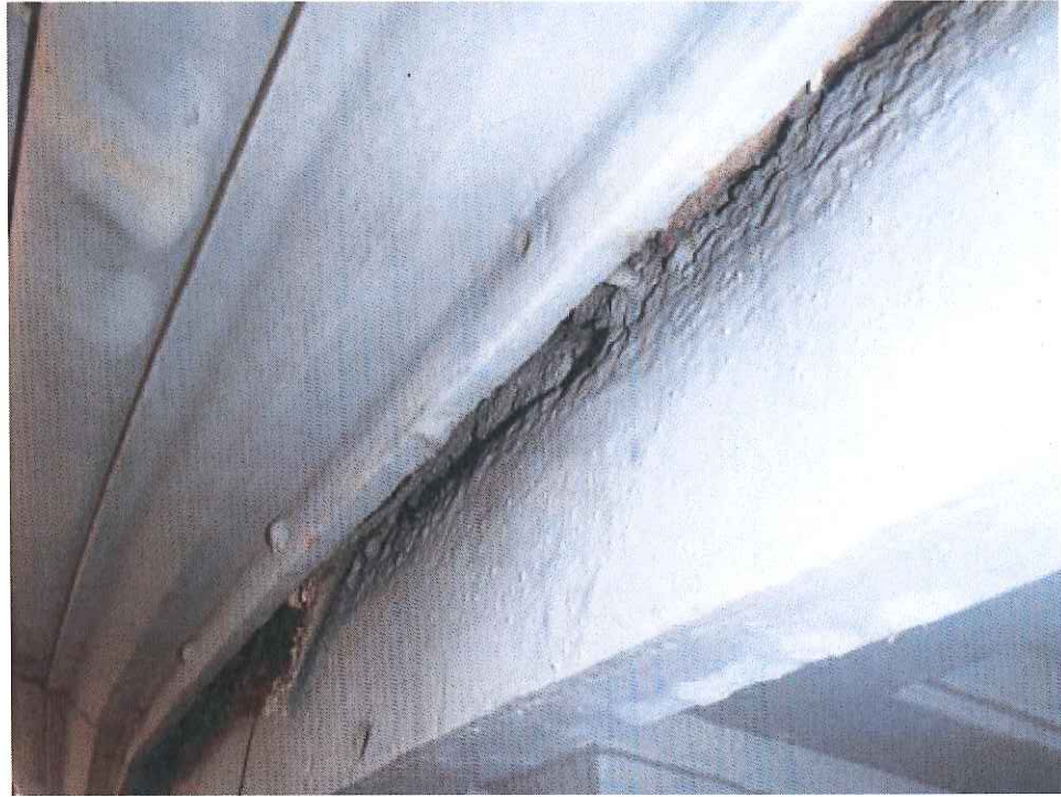
Photo 1.6a: Gutter profile pulling away from vertical plate.
