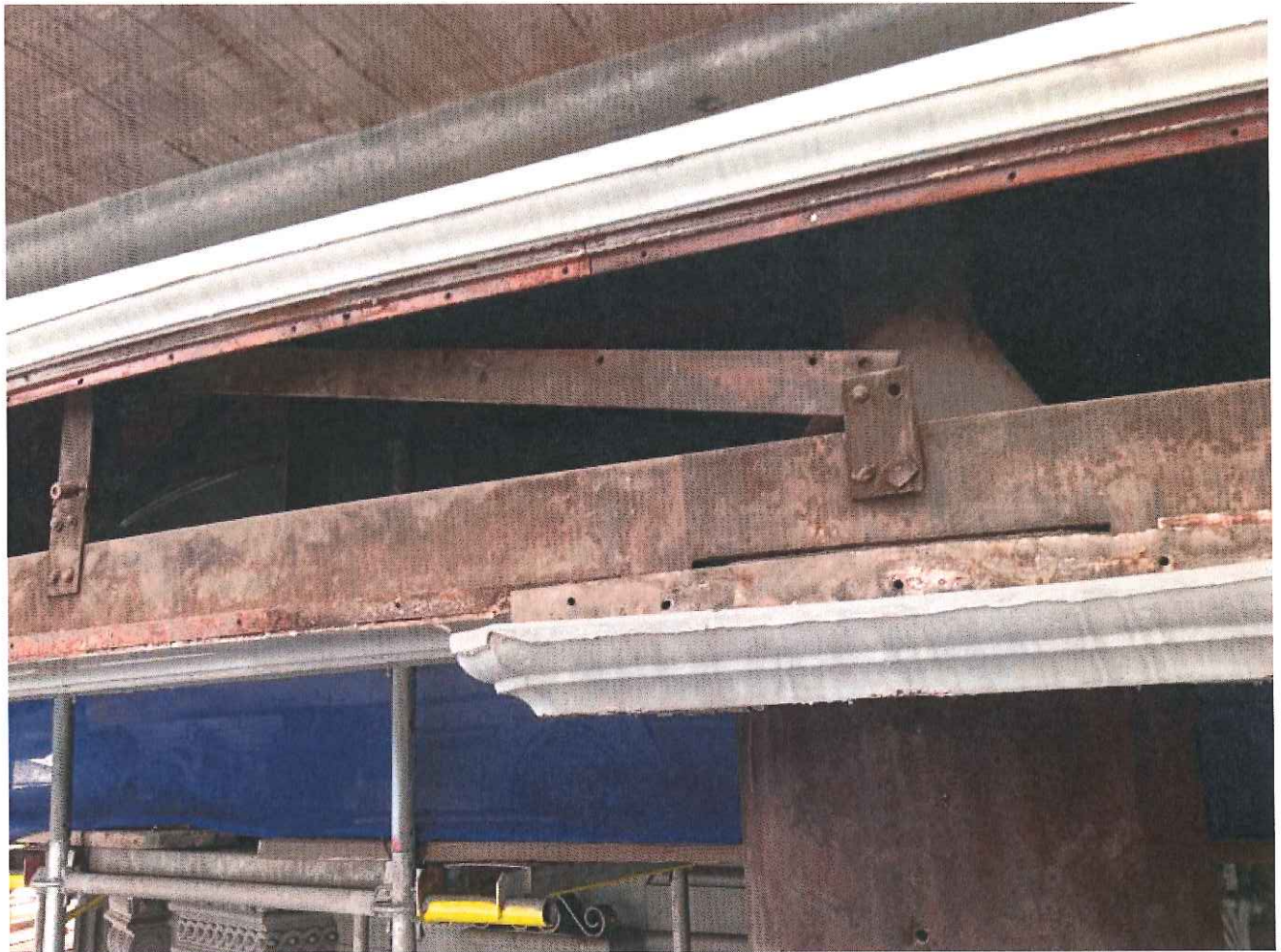
Photo 09.2: Disconnected hanger at grid line C
