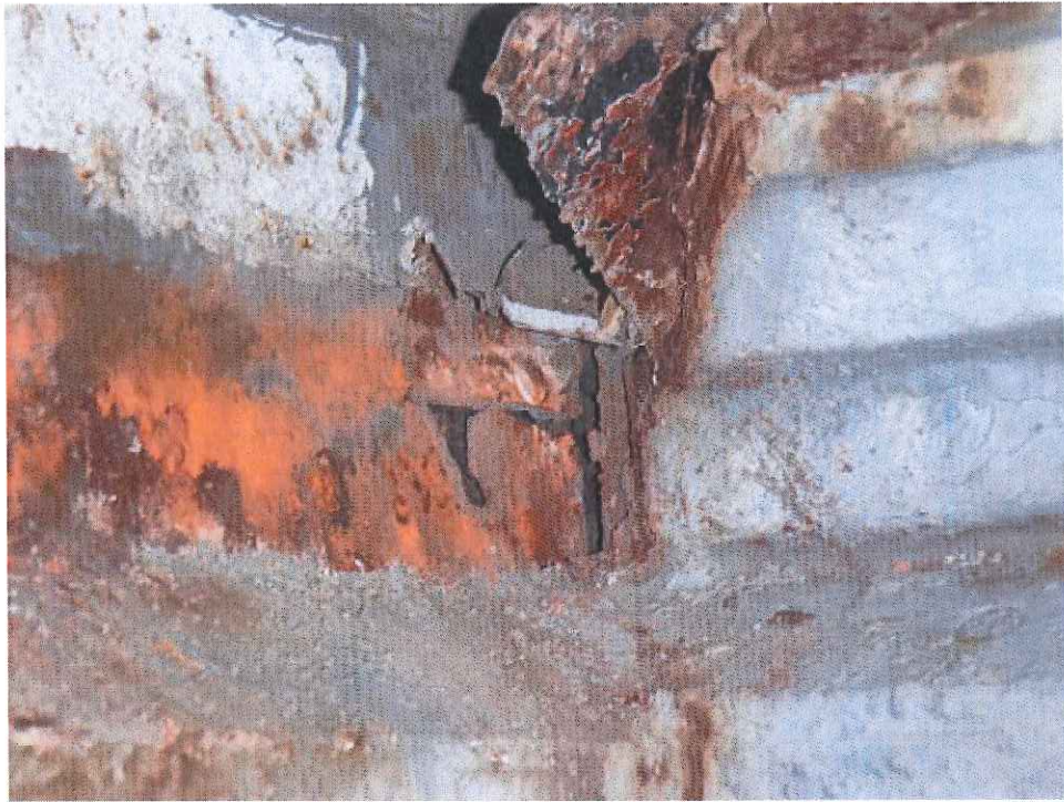
Photo 1.6c: Material loss in vertical plate behind gutter.
