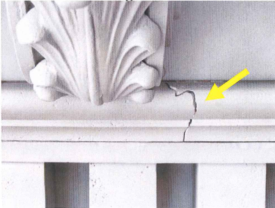
Photo 07.3c: Crack in piece LD-E-10
