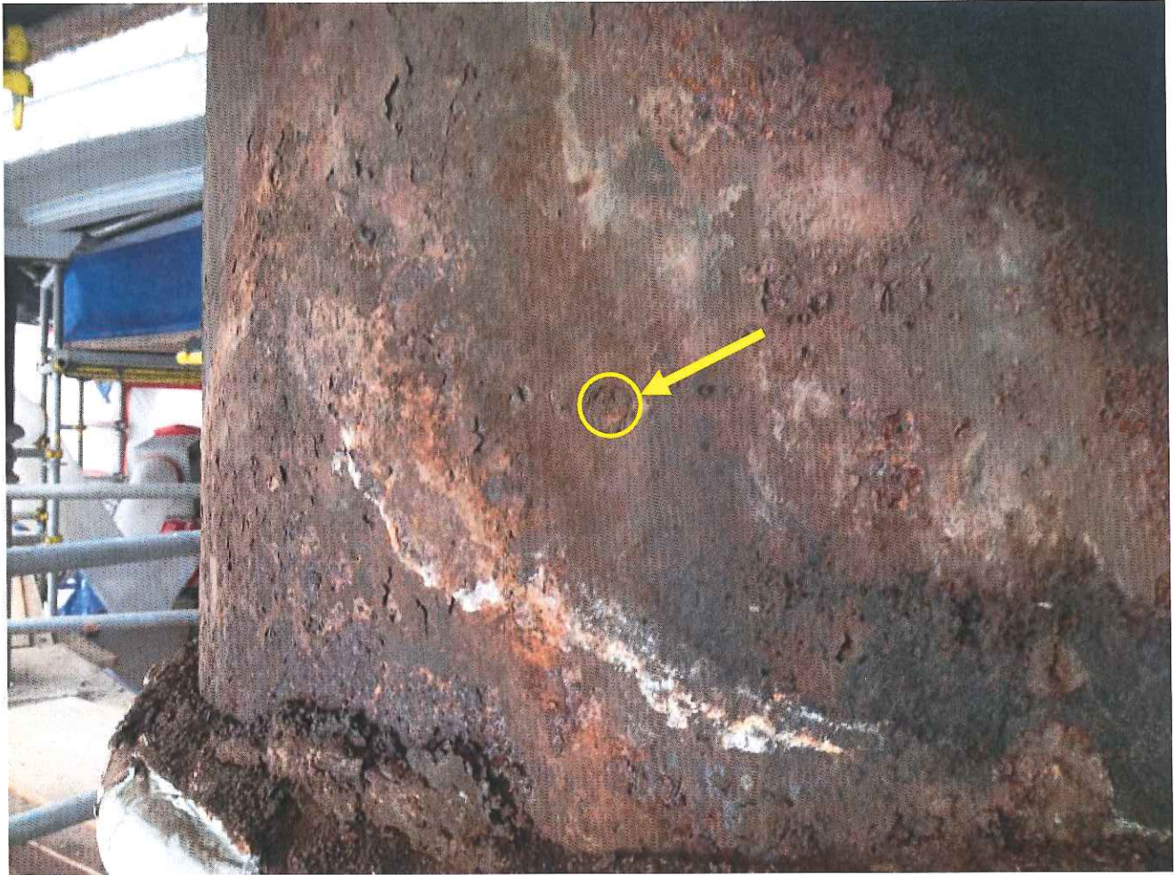
Photo 09.3: Broken bolt to capital on outer column on grid line E
